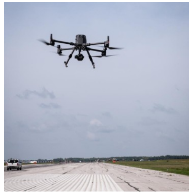
Figure 3. The drone is filming the crack
